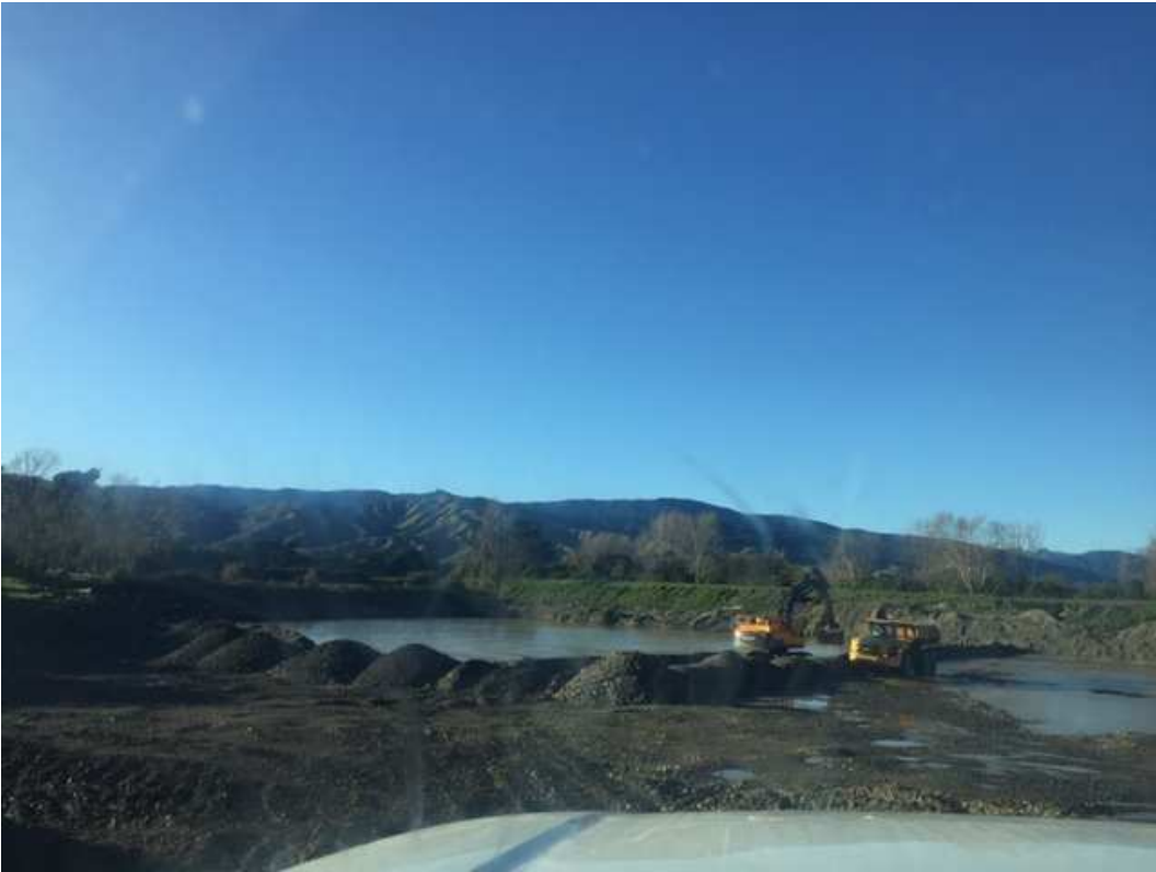
Figure 2: Excavation occurring on Stage 2B. Bank is starting to be stabilised in far corner away from active works (to avoid topsoil being eroded into lake).
